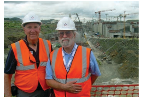
NCS members Bernie Dennis (left) and L.J. Sauter pose at construction of the new Pacific Lock.
