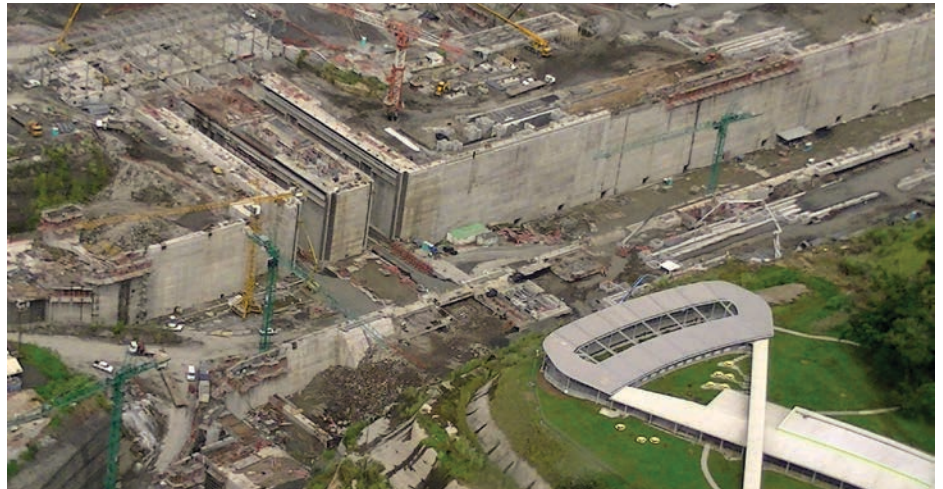
Aerial view of construction at the new Atlantic Lock. Note the two "slot" cuts perpendicular to the canal wall. These "slots" will hold the new rolling lock gates which will block the canal at this end. Another set will be located at the far right – outside the photo – to block the northern end of the lock. Photo by Ernesto Guevara Ortiz, M.ASCE.
